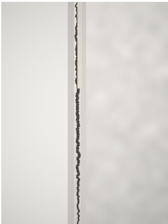
Gap where the sealant run stops
