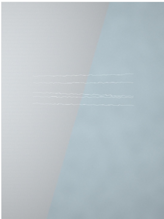
Scratches across the balustrade panel
