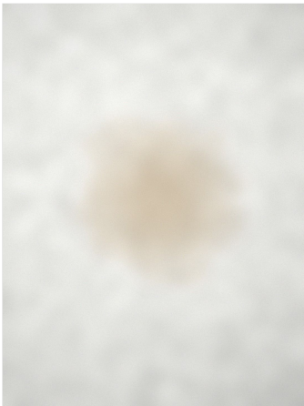
Staining below the level 3 wet area
